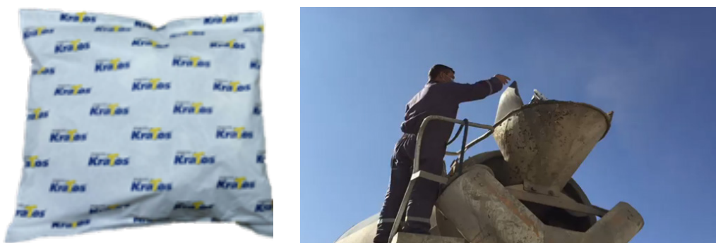
Figure 2. Water Soluble Packages of KraTos Macrofibers and Microfibers and Adding Process on Truck Mixer
